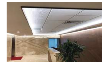
LED energy-saving lighting equipment Settings
