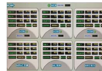
Set electricity environment control system Settings
