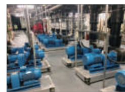
▲ Set up efficient water pumps
